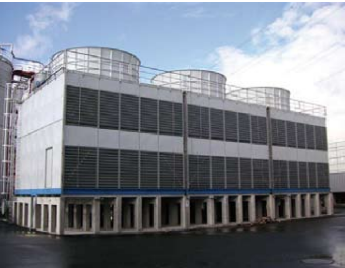
Cooling Tower type 3 XM 2.2.720 Chemical plant in Germany
