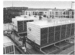
XT cooling tower
